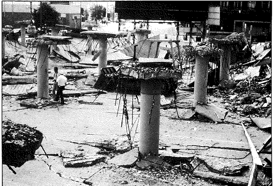
A parking structure which collapsed due to deterioration
