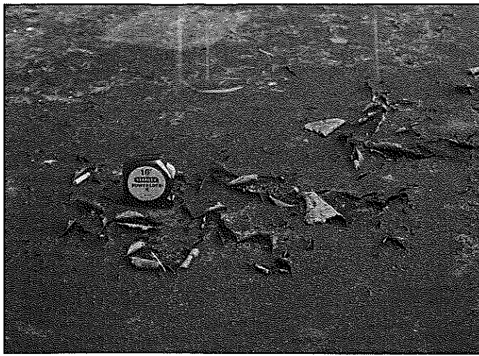
FIRE RESISTIVE coating peeled and delaminated from this single ply membrane in an area of standing water.
