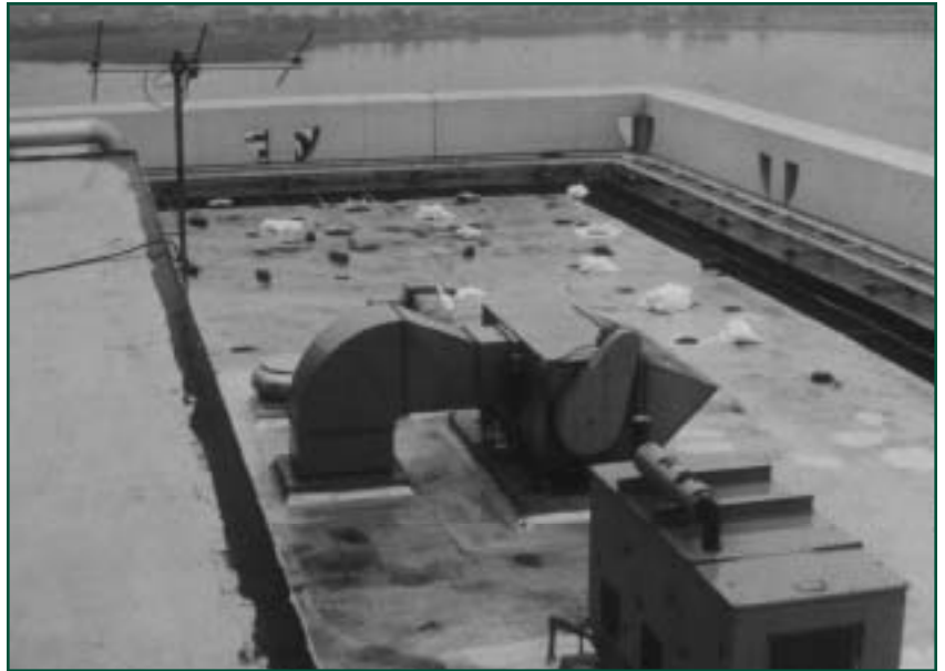
Figure 5: A twelve-story office building that experienced wind damage at wind speeds well below design levels
