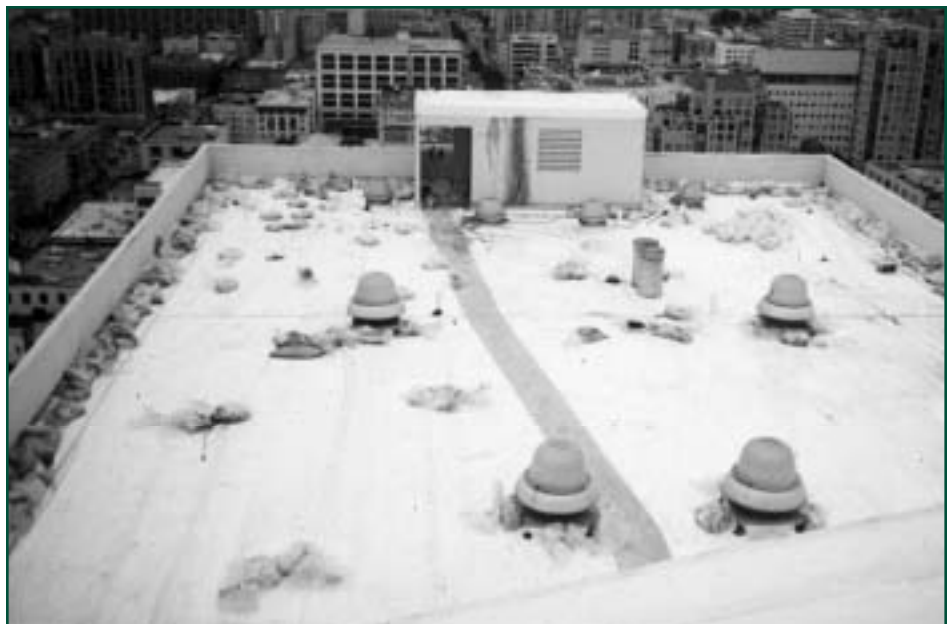
Figure 6: A fourteen-story building with a concrete deck and a fully-adhered, felt-back PVC membrane surrounded by 4' parapet walls that experienced wind damage shortly after installation.
