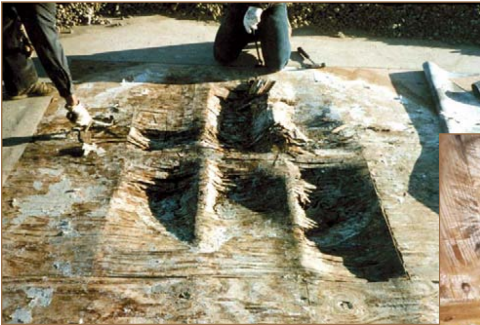
Photos 7 (left) and 8 (below) – Severe plywood deck deterioration with fungi growth caused by condensation over a laundry room in multi-family apartment building.
