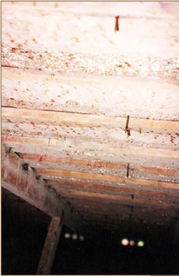
Photos 3 (left) and 4 (below) – Literally thousands of water droplets form on the underside of a plywood and spaced sheathing roof deck despite conventional attic eave vents on a project where a self-adhered membrane underlayment was installed as part of a roof replacement project.
